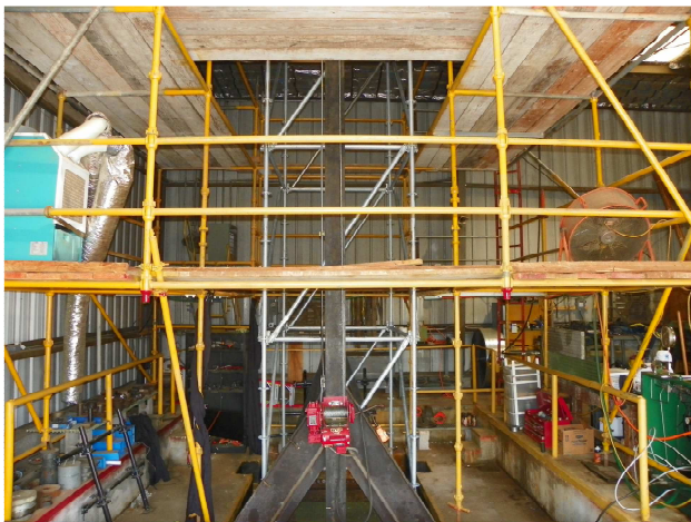
View of Three Tier Tower, before loading
